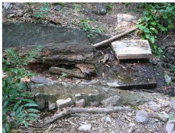
Spring water intake facility in the city of Nueva Esparta (not properly maintained)
