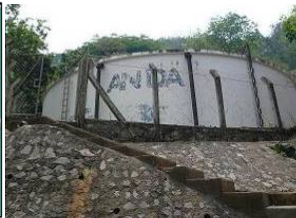
Chinameca Water Storage tank (May 2008)
