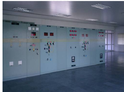
Sub-station Control Room
