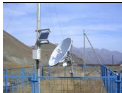
Satellite communication system installed at Thuash tunnel
