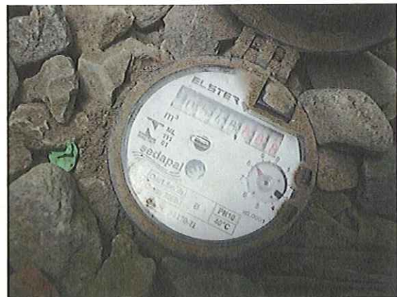
Water meter of SEDAPAL
