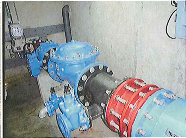
Remotely controlled water distribution valve
