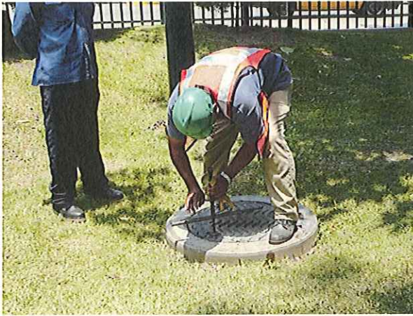
Manhole for the underground water distribution valve chamber at a public park
