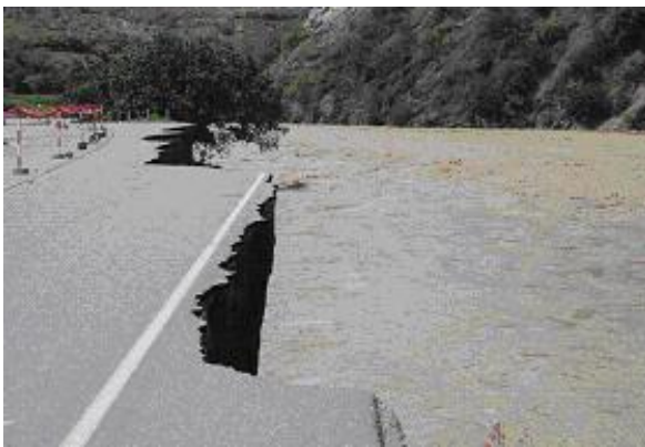
Road Eroded by a River (Olmos-Corral Quemado Highway)
