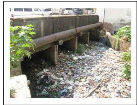
Drainages with garbage (Open drainage in Serpentine area)
