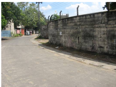
Open side drains with slab lids for easy operation and maintenance (Attidiya)
