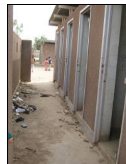
Photo 9 Filthy Latrine Building
