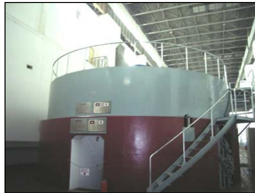
Water Turbine Generator (Unit No. 1)
