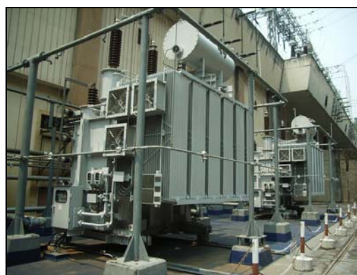
Photo 2: Main Transformers (the Unit No. 1)
