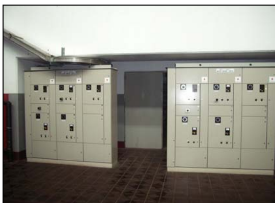
Photo 1: Motor Control Center
