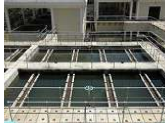
Malimboda Water Treatment Plant (sedimentation pond)
