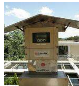
Inlet flow meter of treatment plant
