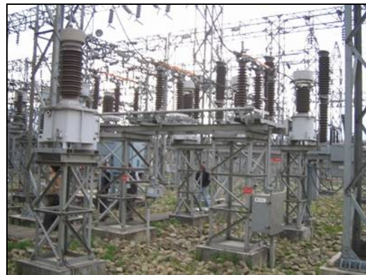
Photo 1: Overview of Equipment in Siuchatar Substation
