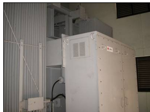
Photo 2: Transformer in K3 Substation
