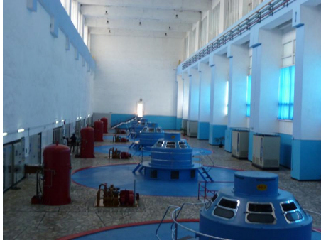
Figure 4: Generator Units (Vau i Dejes Hydropower Station)
