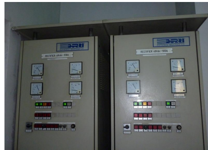
Figure 7: Electrical Equipment Rehabilitated by JICA Loan (Vau i Dejes Hydropower Station)
