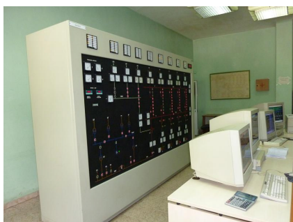
Figure 8: Control Room (Fierza Hydropower Station)
