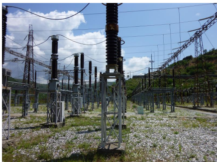
Figure 2: 220KV Isolator Switches (Fierza Hydropower Station)
