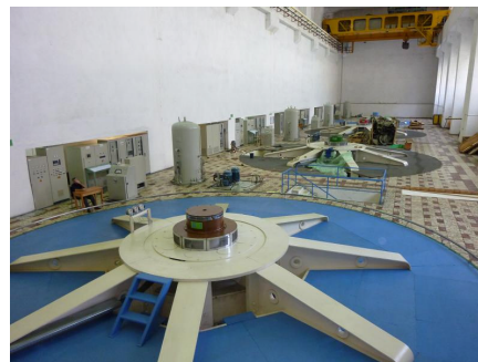
Figure 3: Generator Units (Fierza Hydropower Station)
