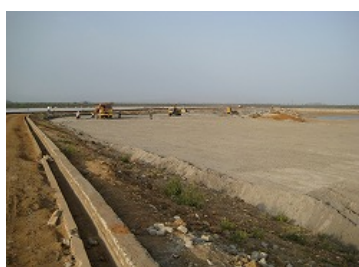
Ash Handling Plant (Ash Dyke)
