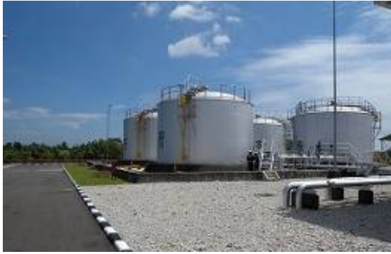
Figure 4 Fuelling System Built by the Project.
