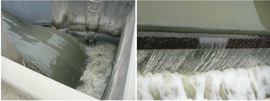
San Bartolo STP : Sewage Inflow before treatment (left), Treated Sewage (right)
