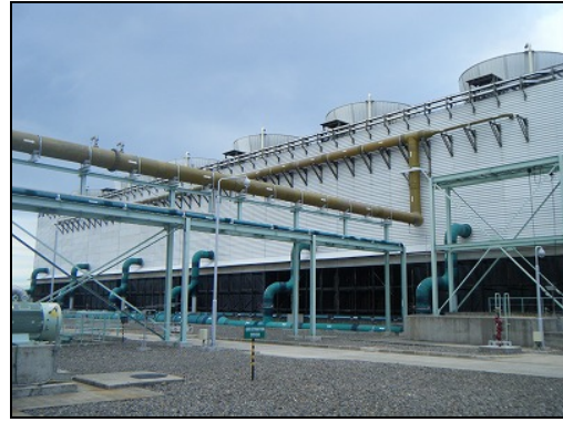
Northern Negros Geothermal Power Plant
