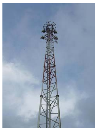
Telecommunication tower of WLL (Suburb of Tunis)
