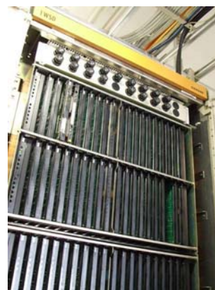
Transmitter (Medjez el Beb station, Béja)
