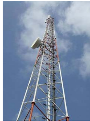
Telecommunication tower of wireless local loops (WLL)
