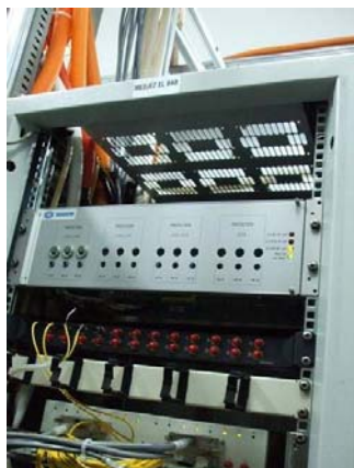
Transmitter (Medjez el Beb station, Béja)
