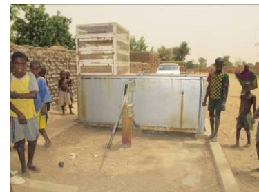
Iron-removal equipment installed along with a borehole with a hand pump (Woroyesso village in Mopti)
