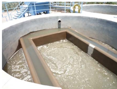
Modified Compact Unit (flocculation and sedimentation basin)
