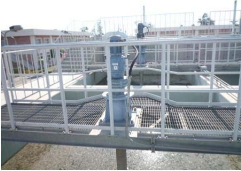
Flocculator (the blue equipment in the middle)
