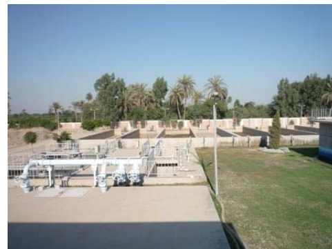
Drainage and Sludge Tanks
