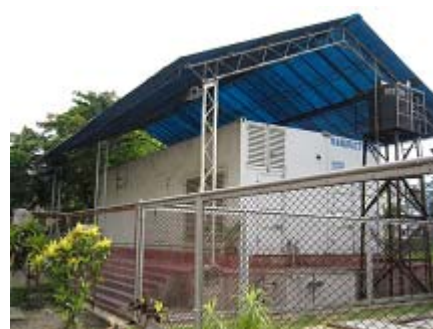
Sewage treatment plant
