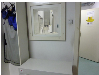
Figure 2: Renovated Monitor Window and X-ray Sealed Door (X-ray Room) (Banja Luka, RS)
