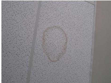
leaks in ceiling
