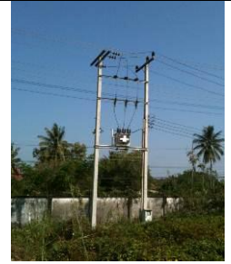
Low voltage 22 kV Transformer
