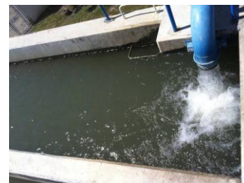
Incoming water holding tank in Cabañas
