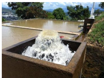
Incoming water distribution system in Sanarate
