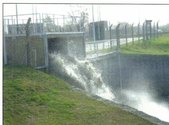
Pump Station No. 9
