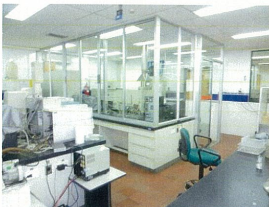
Photograph 1 Water Quality Monitoring Equipment at the Wastewater Treatment Plant
