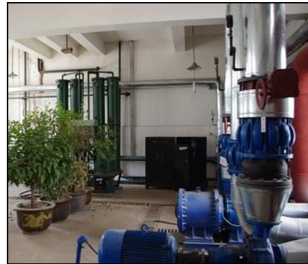
Fig.5 Heat Provision Project Central Heat Provision Facility
