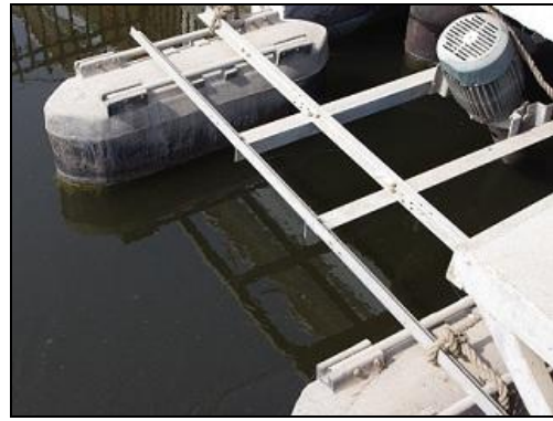
Fig.3 Water Discharged After Treatment
