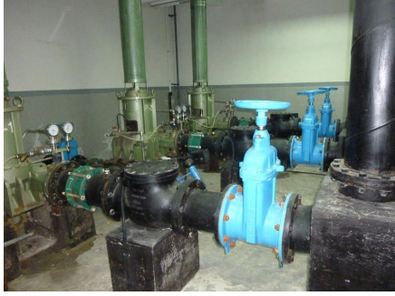
Figure 6: Booster (relay) Pump Station (Sanur Area)
