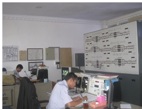
CTC equipment (the central control room at Yogyakarta Station)
