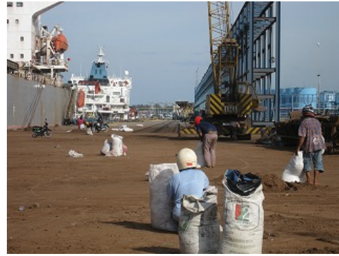
Extended part of the multipurpose wharf after unloading of palm kernel shell (livestock feed). The Phase I project output is in back.
