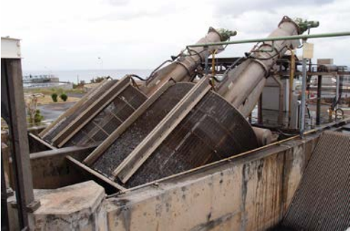
Treatment Plant: Pond (Upper Right) and Trash Filter (Lower Right)
