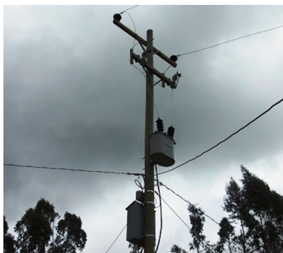
Electric Pole and Transformer in a Rural Area (Cajamarca)
