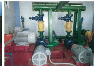
Pinaungon Pumping Station
