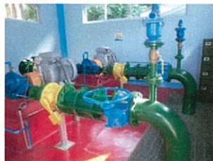
Upgraded equipment in facilities Bolabog Pumping Station
