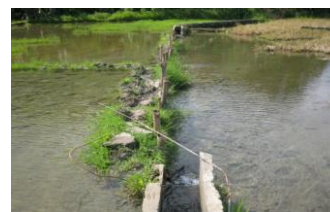
Figure 4: Partly damaged line canal
