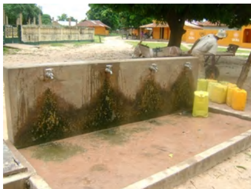
Public water tap in Fass
