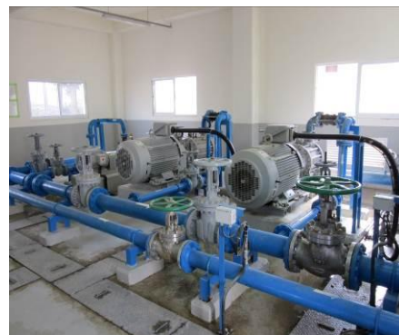
Adasiya Pumping Station
