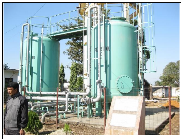
Clear water tank at the Gauradaha Water Purification Plant
