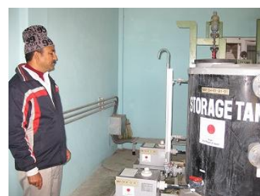
Mangadh Water Purification Plant (sterilizer)
