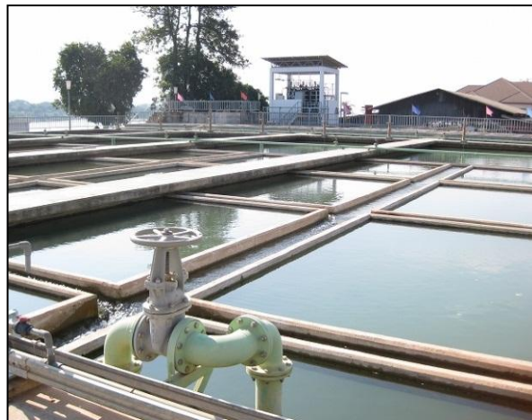
Water receiving well at the Kaolieo Water Purification Plant
