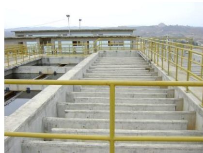
Water treatment plant built by the project
