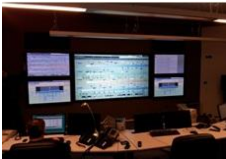
Monitor of SCADA System
