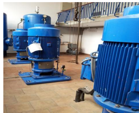
The pump installed in PS 15 by the project
