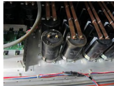
Damaged discharge switch
