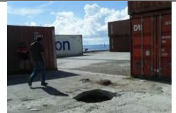
Cavings identified at the container yard
