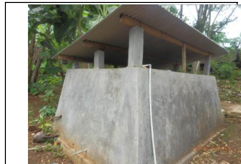
Photo: Common reservoir tank used by the inhabitants. Water supplied from PDAM is stored through pipes and rainwater and tap water are mixed there and used.
