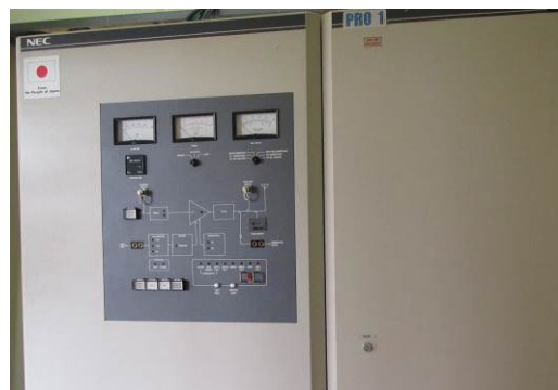
Transmitter Equipment for medium wave radio
