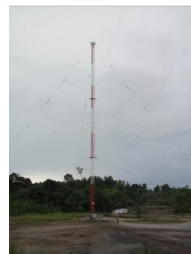
Medium wave transmission antenna
