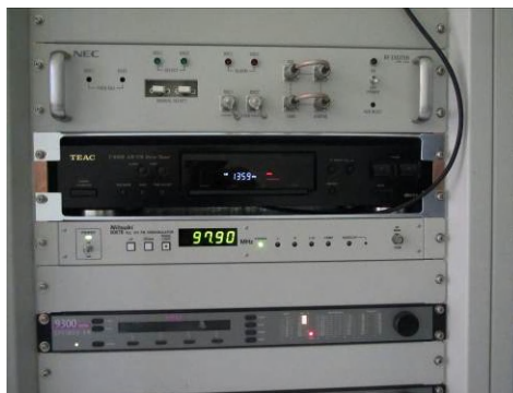
Program input/monitoring equipment
