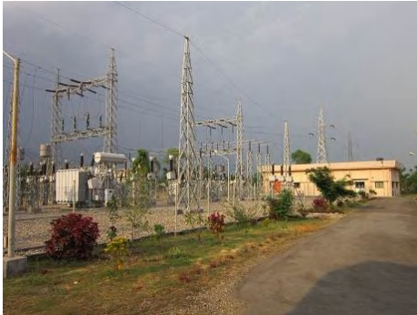
External View of New Kawasoti Substation
