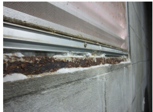
Photo: A window sash on which salt is deposited because wind brings salt
