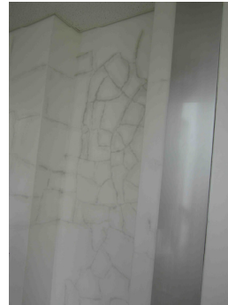
(Cracks after repairs at the Subang DIC)
