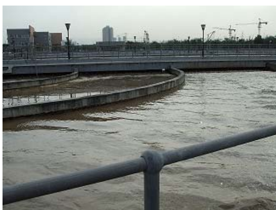
No.3 Wastewater Treatment Plant (Orbal oxidation ditch)
