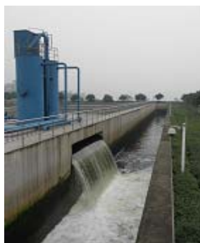
Wastewater Outlet of Juguanshi WWTP
