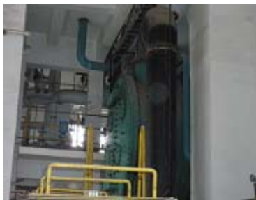
Turbine of the remaining heat supply system
