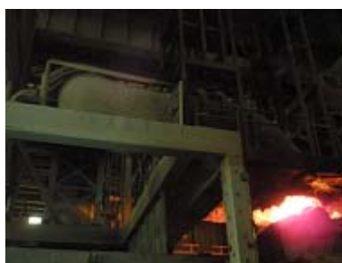
AOD furnace and dust remover
