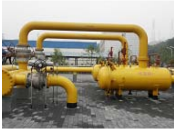
Filtration machine at Toutong Gas Storage Station
