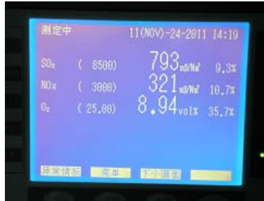
Waste air monitoring equipment at Chongqing Power Plant
