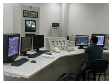
Central control room
